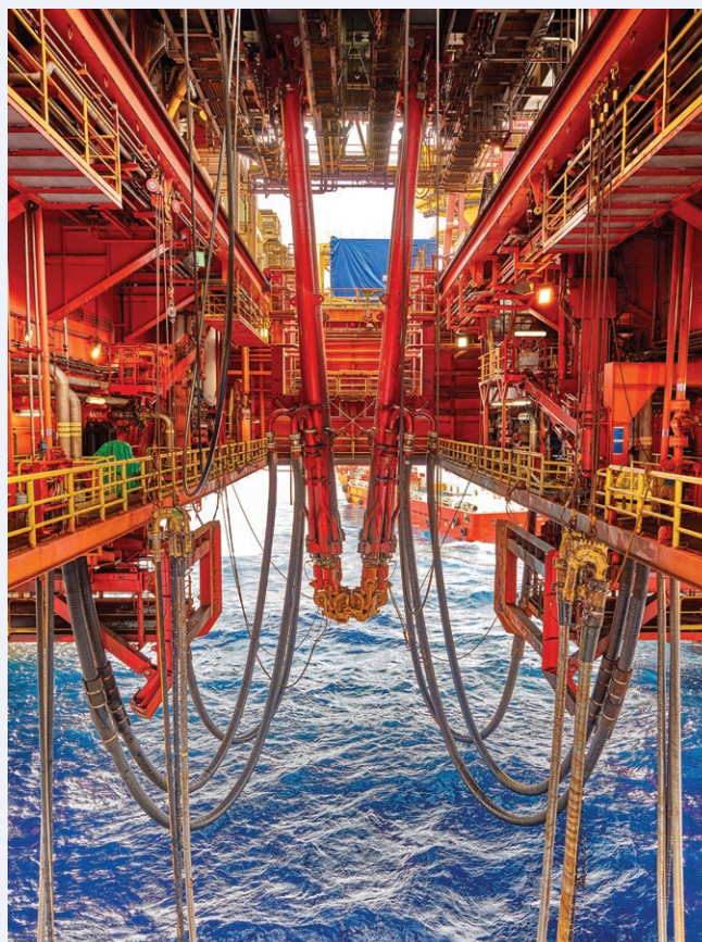
Construction at the Lihua 29-1 field at the Liwan Gas Project is progressing with first gas production set for the fourth quarter of 2020.
