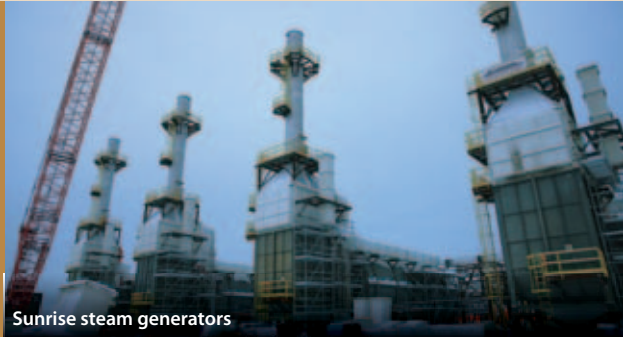
Sunrise steam generators
